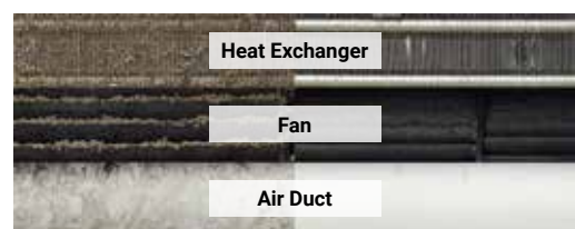
Without Dual Barrier Coating (After 10 Years) With Dual Barrier Coating
